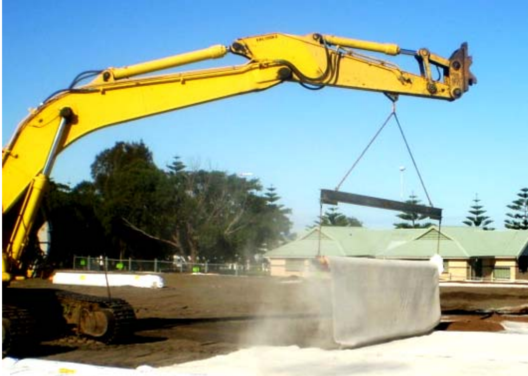
FIGURE 1 – LOSS OF POWDERED BENTONITE DURING GCL DEPLOYMENT
